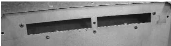
Fig 4 - Flue Restrictor Baffle Not Fitted
