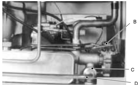
fig. 69 (rear view of the boiler)
