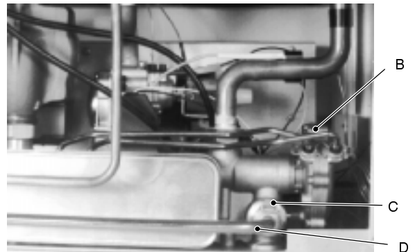
fig. 70 (rear view of the boiler)
