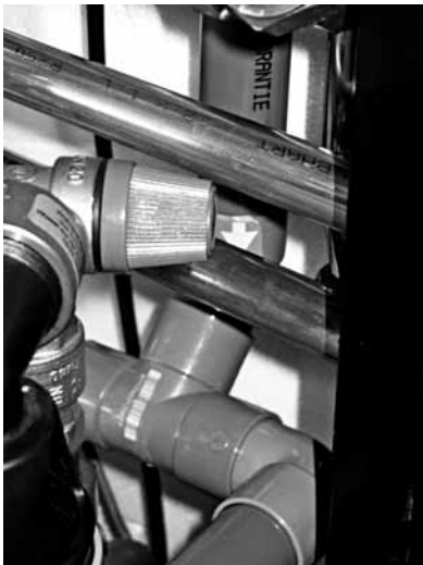
Condensation drain pipe
